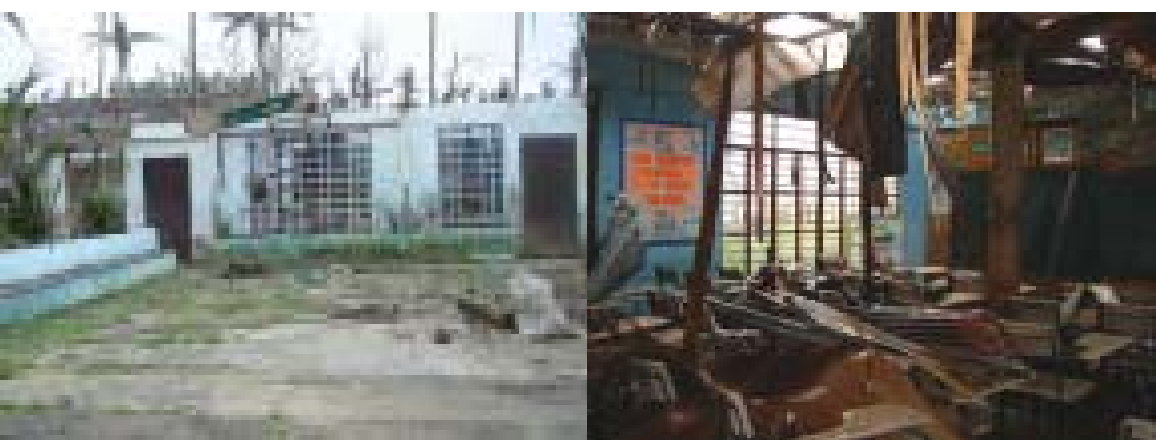
Damaged School Buildings
